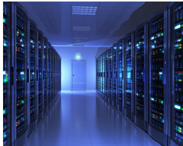
Data Center Solutions
